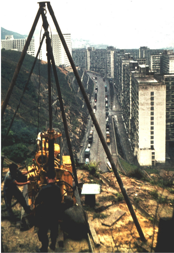
Figure 11: Drilling vertical diamond core holes into the Sau Mau Ping slope. These holes were used for geotechnical investigation purposes and also for the installation of piezometers in the rock mass.
