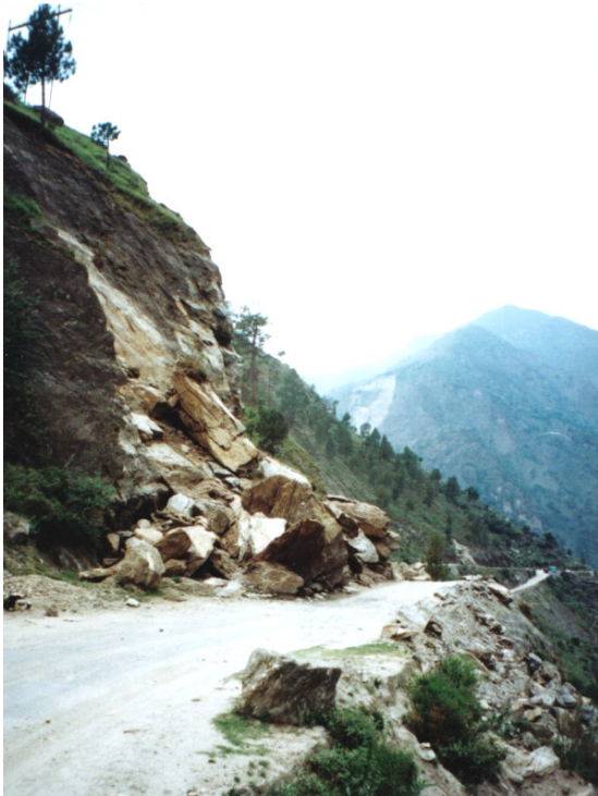
Figure 3: A rock slide on a road caused by the undercutting of sheet joints in a granite slope. In hard rocks such as granite, failure can occur very suddenly if the factor of safety of the slope is close to 1. A rise in groundwater levels during a heavy storm or ice jacking in winter may be sufficient to induce failure.
